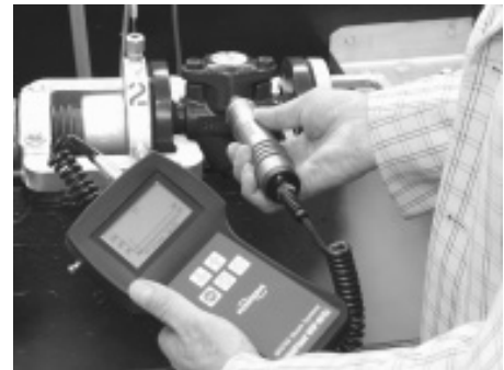
Checking steam trap
